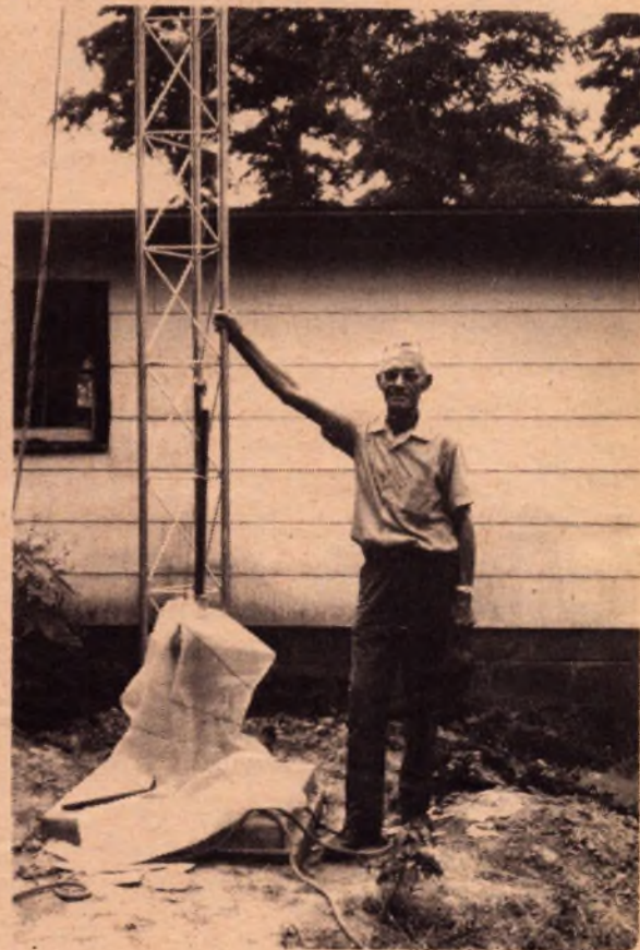
The photo shows Ray erecting a 50 ft. tower for club station WA8LEI at The Grail, Loveland, Ohio.
