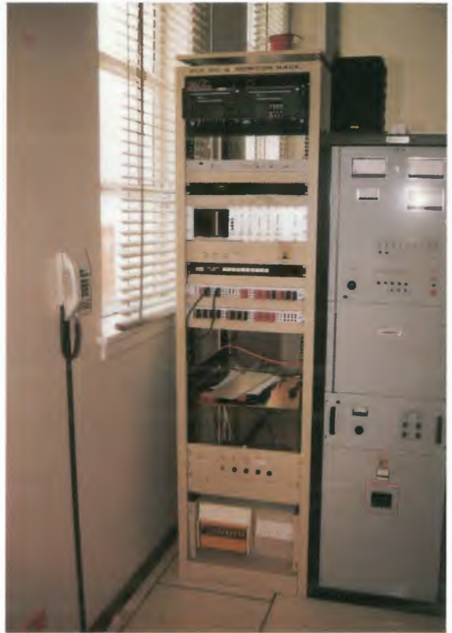
New PIE and PLC Controller.
