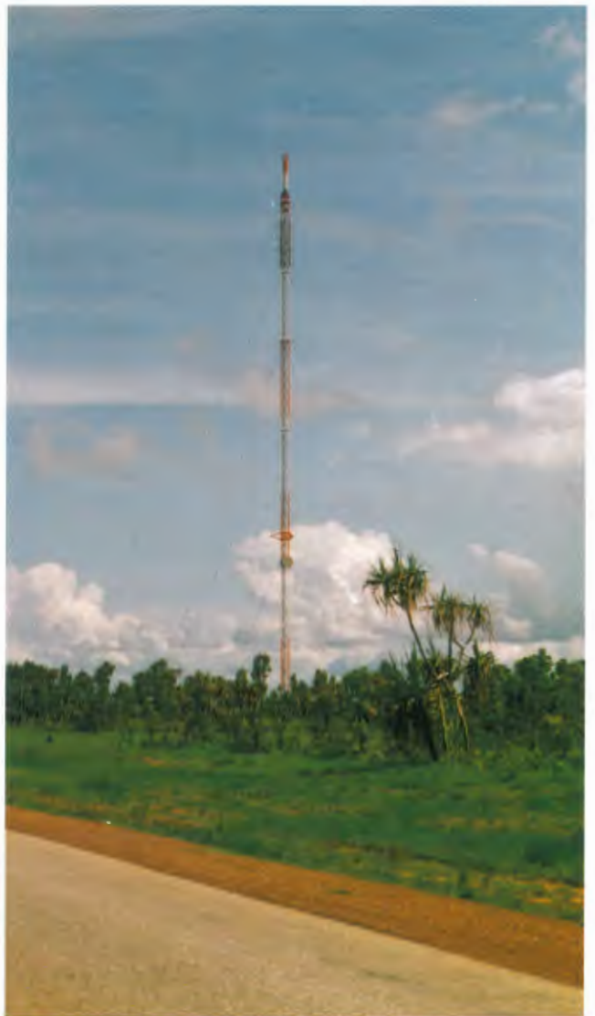
Completed 130 metre mast with antenna systems.
