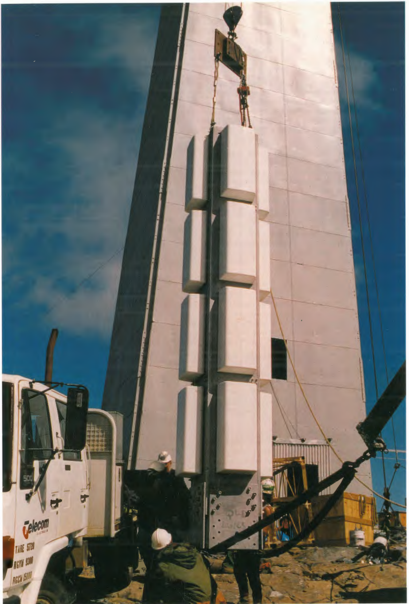
Preparing to lift the bottom UHF module during Mt Barrow upgrade project.
