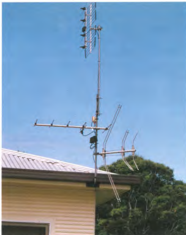
UHF phased array, horizontally polarised Yagi and broadband VHF antenna.
