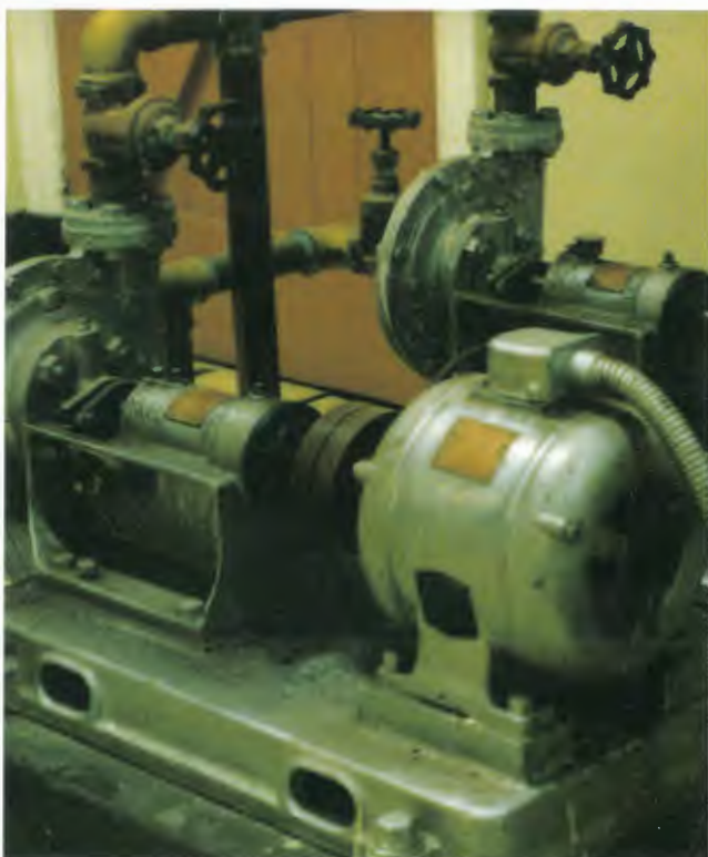
Water pump system original VLQ installed 1943.
