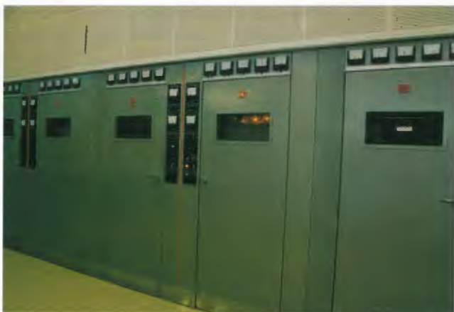
VLW 10 kW STC type transmitter installed 1962/63.
