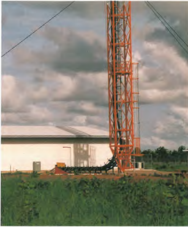
Cable tray for cable access to building.
