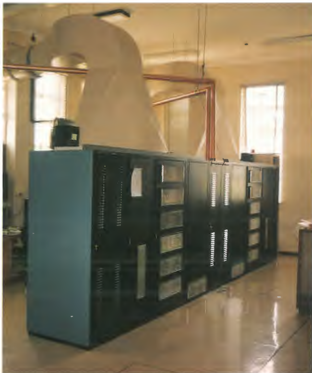
Nautel 50 kW transmitter.
