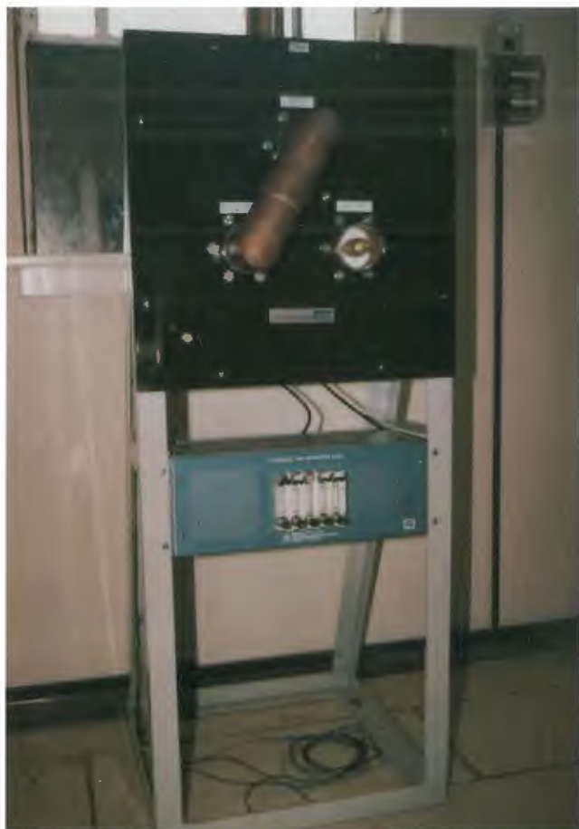
Antenna and load patch panel.
