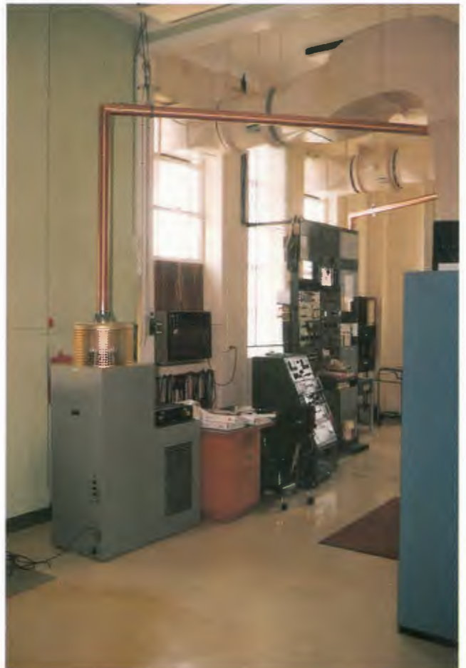
Transmitter load, instrument cart, old PIE and transmitter duct system.
