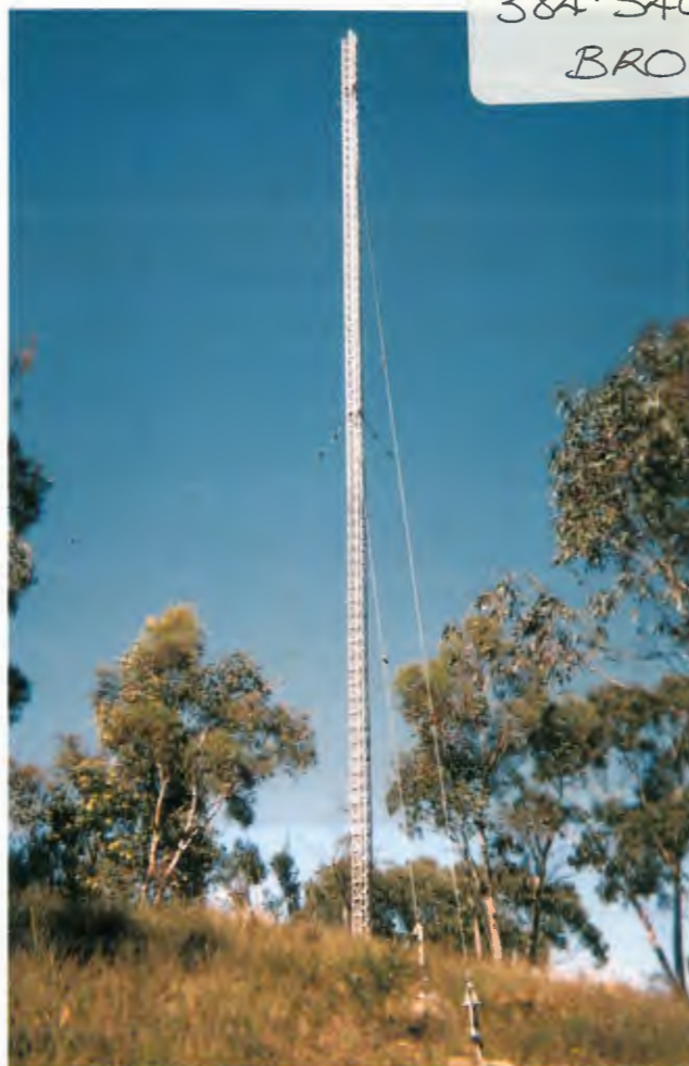
Lattice steel radiator installed on hill above transmitter building.
