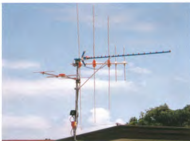
UHF Yagi, VHF Yagi and wideband vertically polarised VHF antennas.
