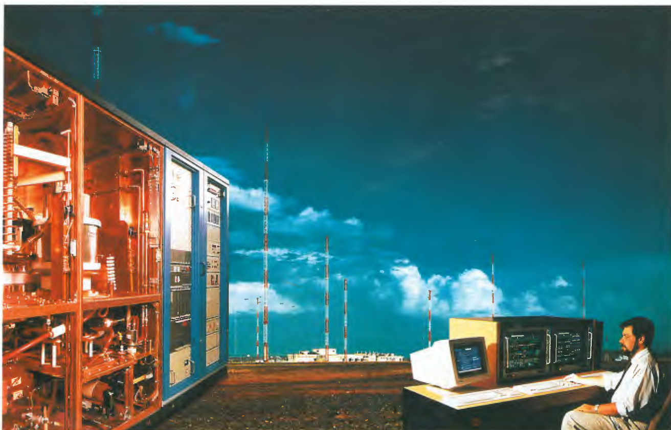
The BROADCASTMASTER control system. (Photo courtesy Asea Brown Boveri)
