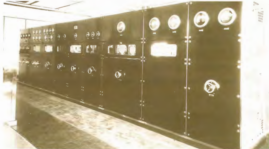
Transmitter installed and operational in Perth.
