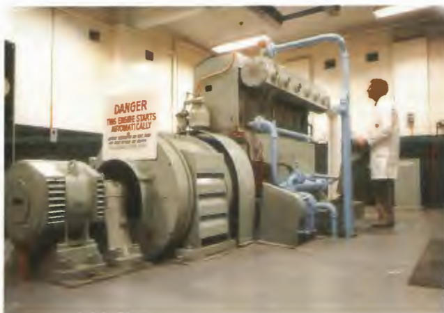
Emergency Power Plant.
