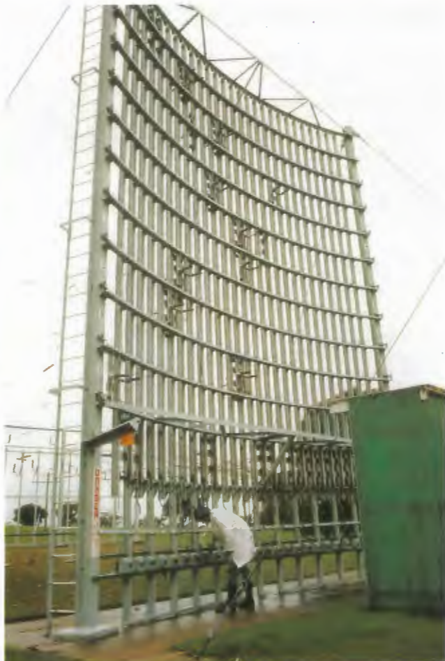
Technician Mark Chapman Operating Line Switch.
