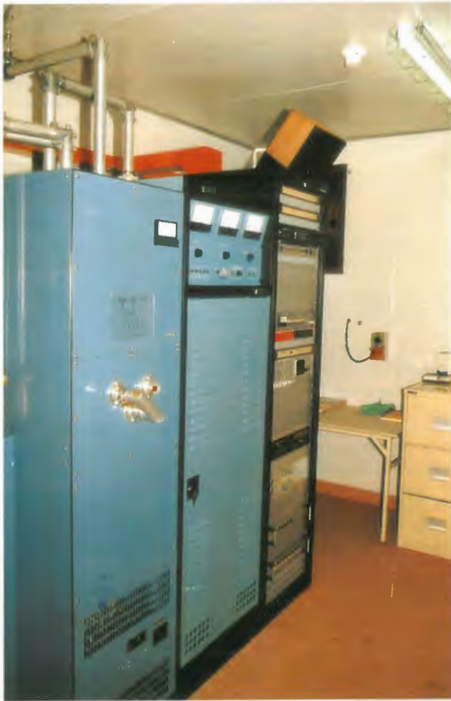
10 kW Nautel Transmitter.
