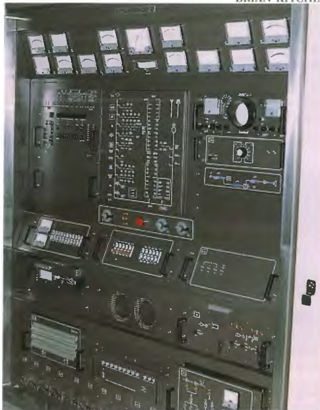
300 kW transmitter front panel.
