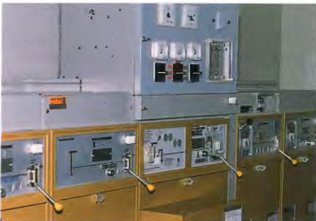
22 kV Distribution unit.
