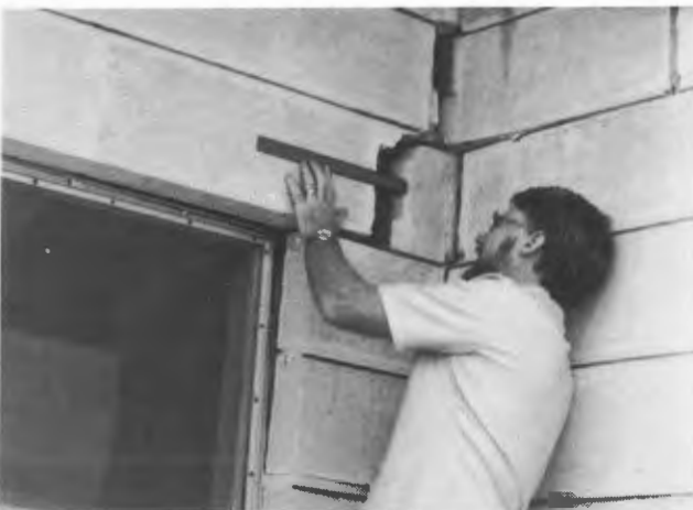
OIC Roger Hedley checking wall movement.
