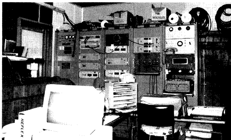
Photo 2 - VK3ZA satellite equipment racks
