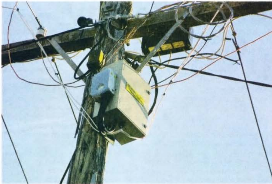
The on-pole BPL repeater hardware.
