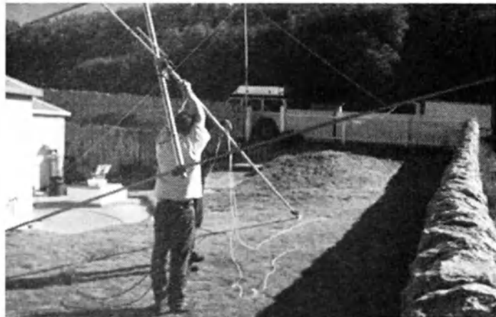
Up it goes! Rhett VK3VHF and Mark VK3MOA preparing to erect a 2 element Triband Yagi 10 m 15 m and 20 m
