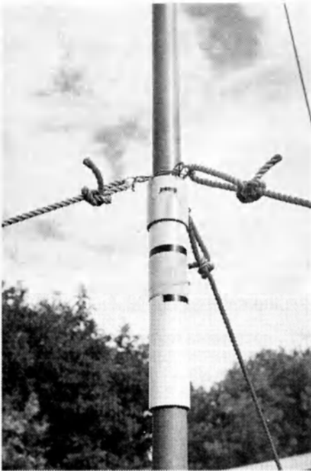
Photo 2 - One of the PVC sleeves showing the attachment of the guy ropes.
