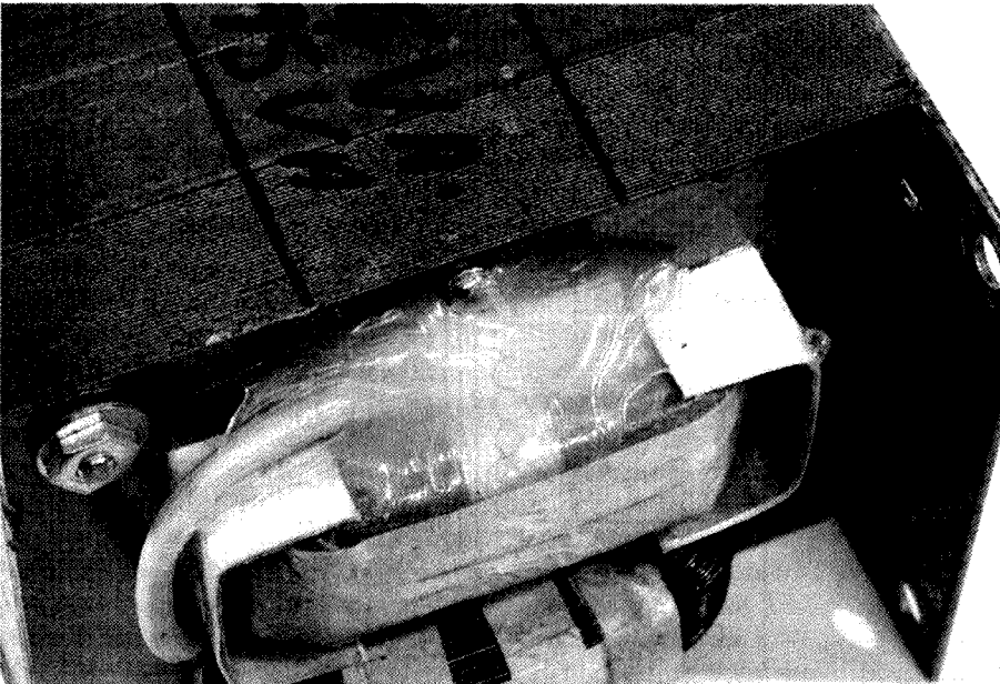
Photo 3 - Siliconed HV wire connection.
