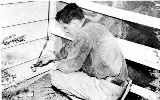
Every detail in the installation is important—note the drip loop which was provided to prevent rain water from entering the building.
