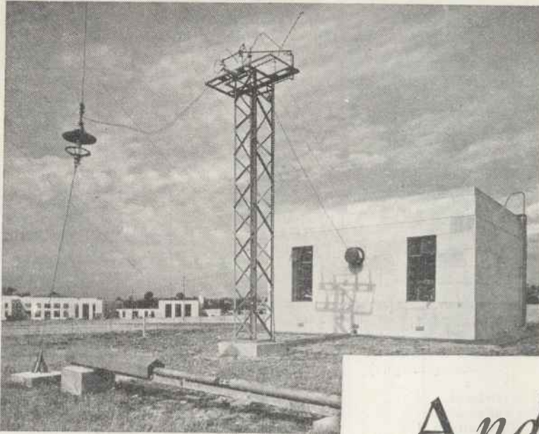
B.B.C. photo This is the aerial-transformer house at Droitwich. The wires from the transmitter are carried on small poles (seen on the left). In the foreground is the aerial-tensioning device which keeps steady the download from the huge Droitwich aerial
