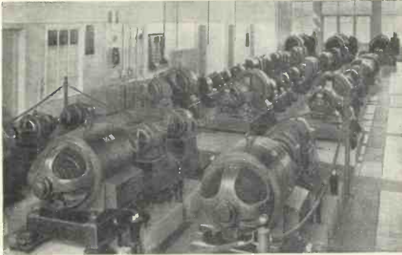
PRODUCING POWER FOR WORLD-WIDE COMMUNICATION Fig. 3.—Machinery hall in Short-wave Transmitter House II
