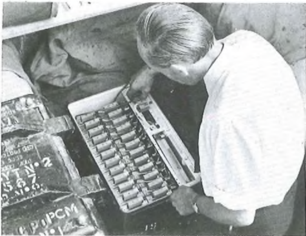
Fig. 4—Installation of a 24-channel PCM system
