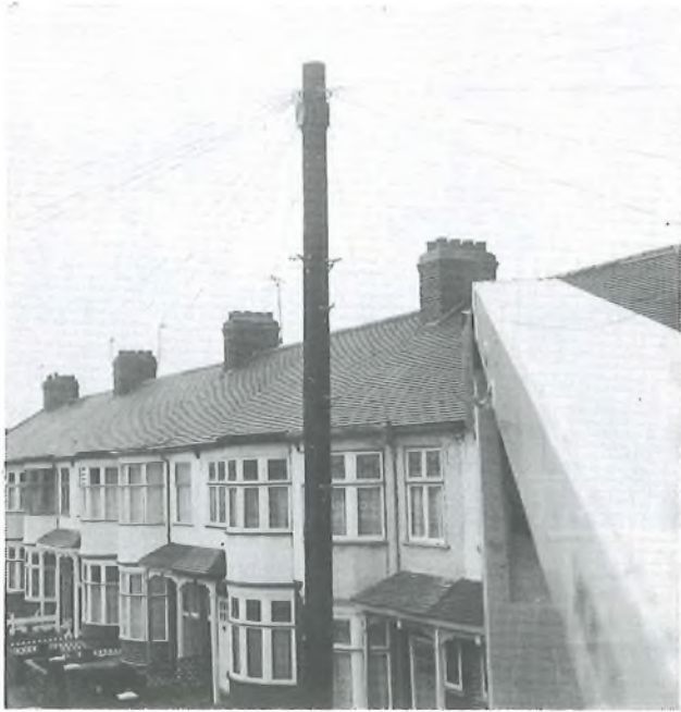
FIG. 12—A modern wood distribution pole
