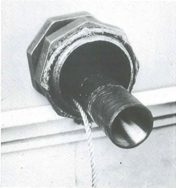
FIG. 11—Millimetric waveguide in its steel duct
