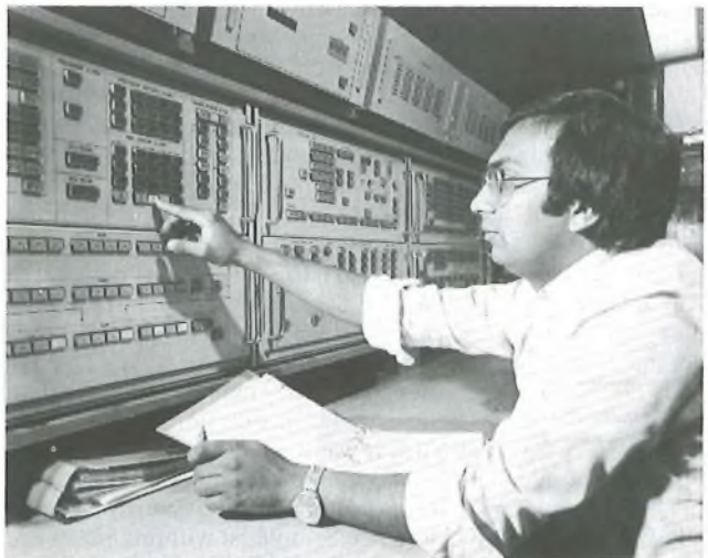
FIG. 11—The Thames ISC TXK6 control room, Mondial House
