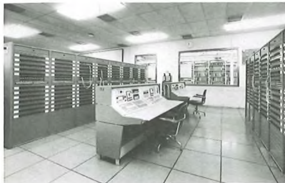
FIG. 7—Part of Mollison ITMC showing test consoles and test-jack frames
