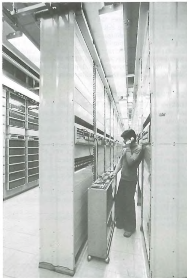
FIG. 5—TXK5 line relay-set and crossbar-switch racks with exchange tester trolley
