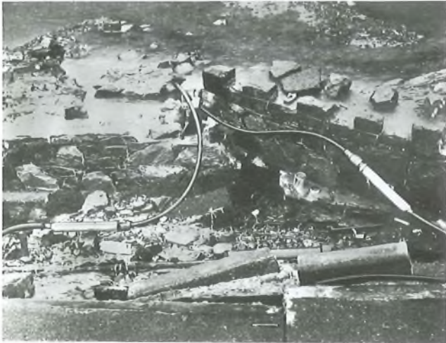
The exposed cables, showing the 3 m length of temporary repair cable jointed in
