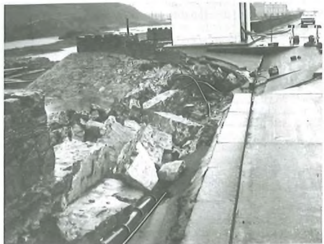
The collapsed sea front at Barmouth
