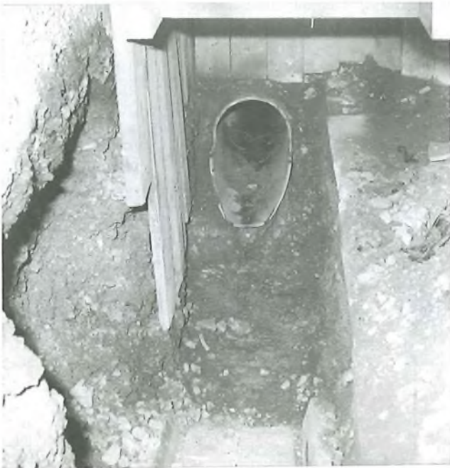
The gas pipe and duct-entry pit
