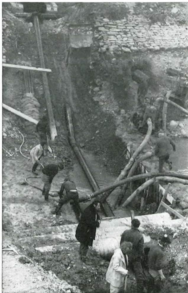
British Post Office duct with sand bag protection on the left and the other two services in position before reinstatement of canal bed and embankments.
