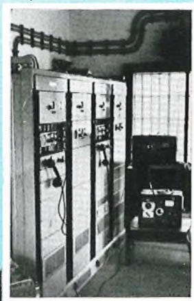
V.H.F. Equipment at Kerewan Repeater Station.
