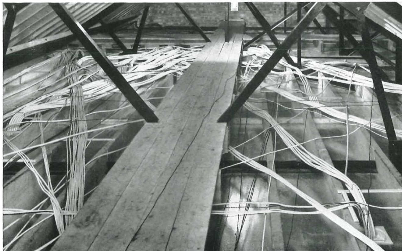
FIG. 1—CABLING ABOVE THE CEILING AT BISHOPS CLEEVE EXCHANGE
