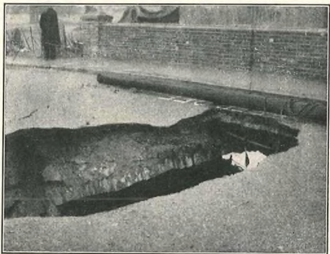
HOLE IN BRIDGE AT HADLOW, SHOWING TEMPORARY SUPPORT FOR ONE POST OFFICE CABLE.
