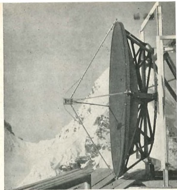
Snow and ice failed to delay the rapid installation of the G.E.C. aerial which faces Chasseral at the Jungfrauoch.
