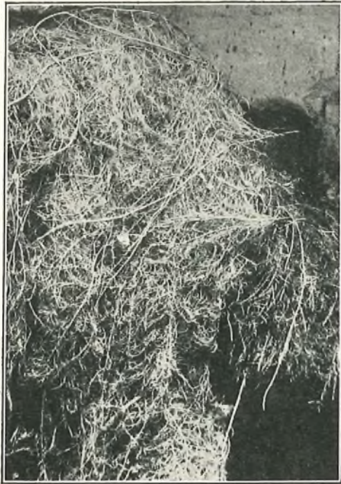
ROOTS GROWING IN MANHOLE.
