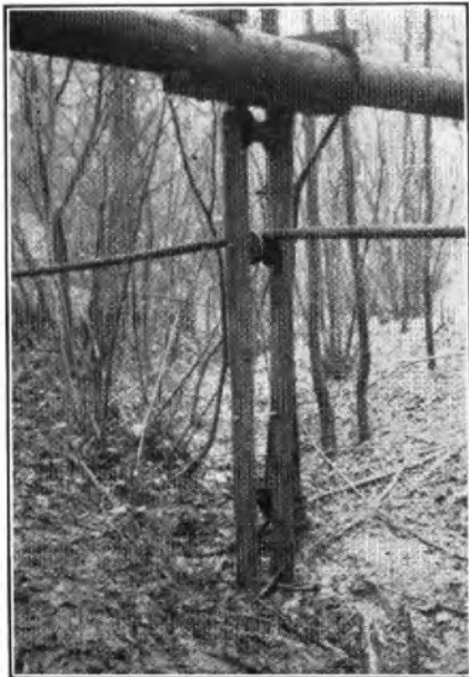
DEVICE TO LIMIT MOVEMENT OF PULLING ROPE AND, LATER, TO SUPPORT WEIGHT OF CABLE.
