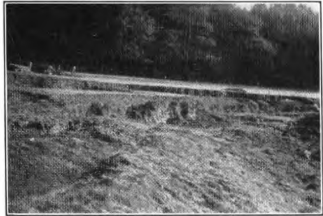
THE EMBANKMENT ONE WEEK AFTER STARTING TO SLIP.
