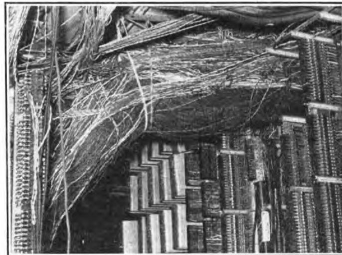
M.D.F. WIRING IN CARDIFF MANUAL EXCHANGE.
