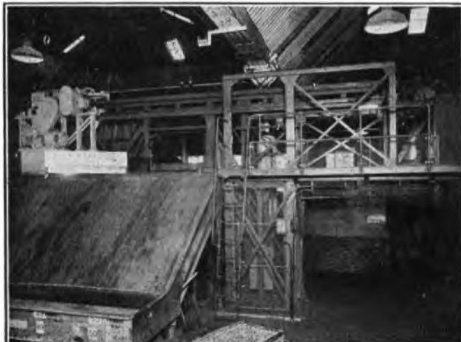
FIG. 4.—THE PLOUGH, GLACIS AND CANTILEVER STRUCTURE ON WHICH THE PLOUGH IS PARKED AND CONTROL GEAR MOUNTED.
