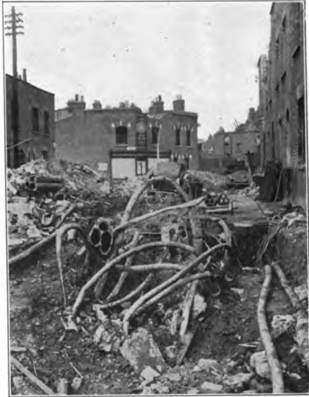
FIG. 2. DAMAGED UNDERGROUND CABLES.
