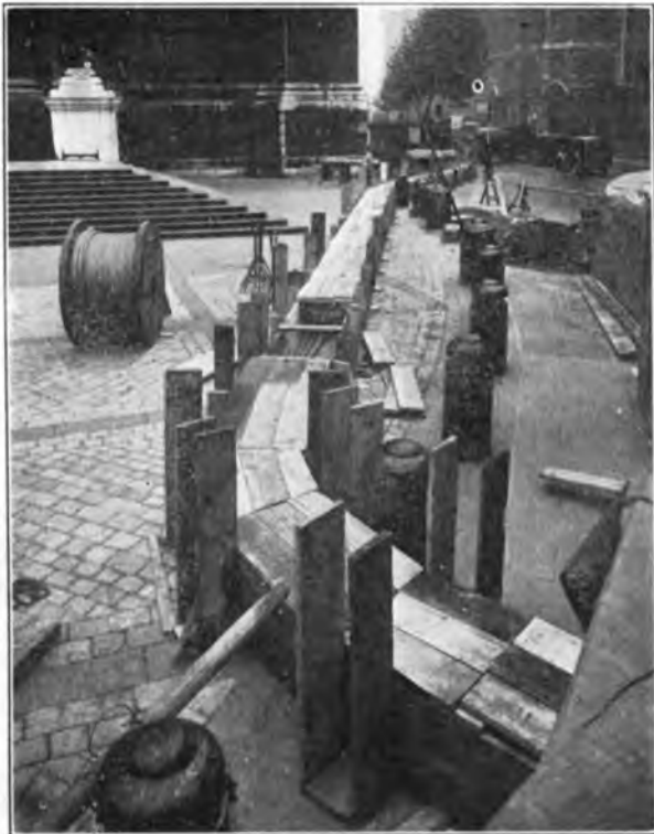
FIG. 5. TEMPORARY CABLE IN TROUGHING.
