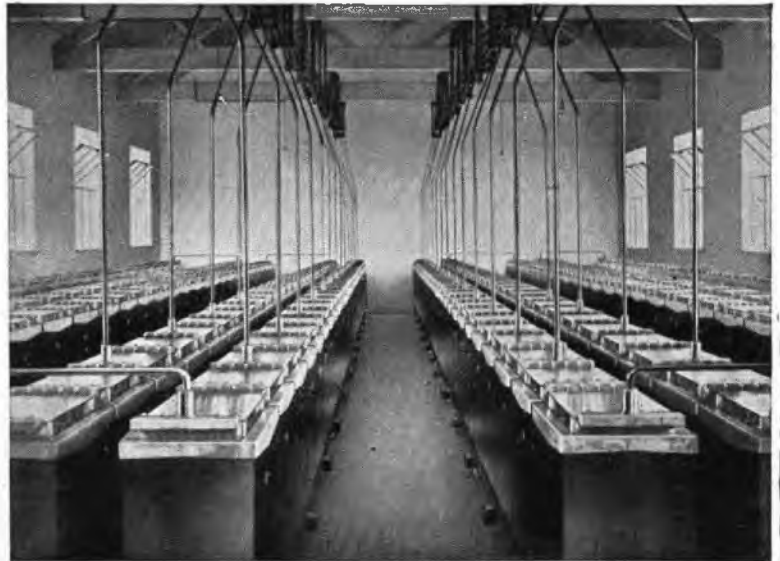
ALTON Battery of 264 DLWII Type Cells at a Corporation Electricity Works
