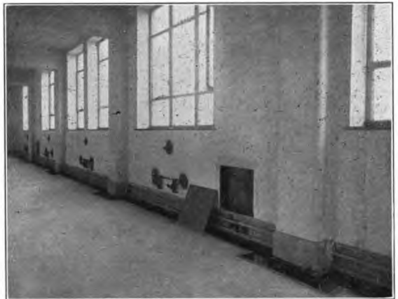
FIG. 2.—STEEL SKIRTING, HEATING PIPE TRENCH AND CONCEALED TELEPHONE SUB-DISTRIBUTION BOARD.
