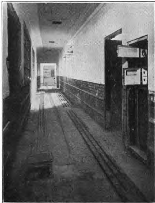
FIG. 1.—ENTRANCES TO MAIN VERTICAL DUCTS, ELECTRIC LIGHTING CONDUIT, AND FEEDS TO UNDERFLOOR DUCT SYSTEM.
