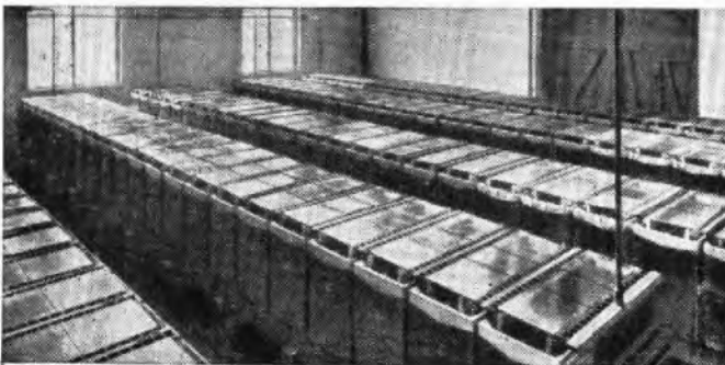
Part of the Alton Battery equipment installed at the B.B.C. Scottish Regional Transmitting Station.
