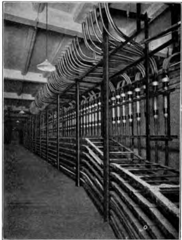
FIG. 3.—THE NEW CABLE CHAMBER.
