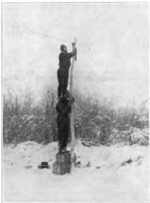
FIXING ONE OF THE INSULATORS OF THE MAIN TELEPHONE LINE TO THE OLD FORT RAE.
