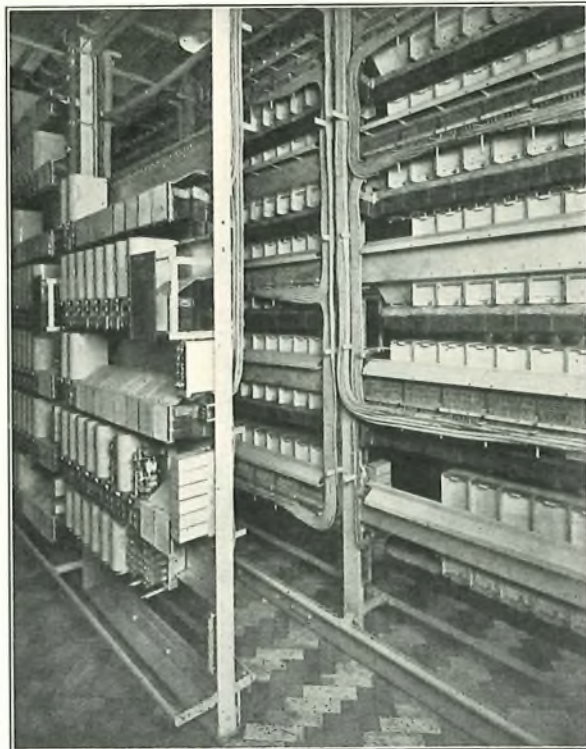
FIG. 3.—SECOND SELECTOR RACK, SHOWING CONTROL RELAY-SETS.
