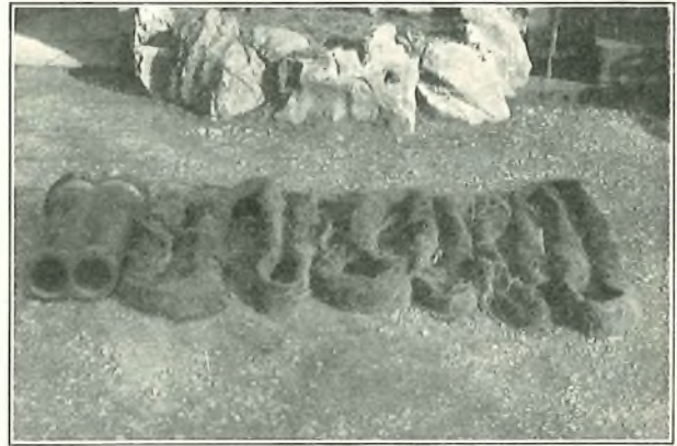
FIG. 1.—PORTIONS OF ROOTS OF DOUGLAS FIR TREE WITHDRAWN FROM 2-WAY DUCT LINE.
