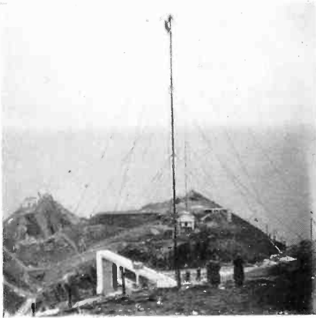
For the guidance of shipping: a Marconi Automatic Wireless Beacon station in course of erection at Mizzen Head, Ireland.
