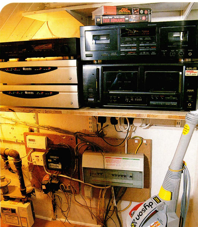
The spaghetti effect of cables and interconnects, can become a thing of the understairs cupboard with a multi-room system. Below-left: B&W's in-wall Casa speakers incorporate amplifiers.
