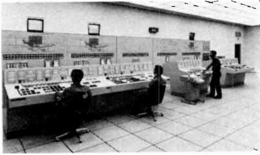
Fig. 5. The control room of the energy-saving refuse incinerator plant at Ulu Pandan, Singapore. The plant will produce low-cost electricity while providing an effective way of disposing of rubbish. Kent were responsible for the instrumentation: BBC Brown Boveri of Mannheim were responsible for the electrical generating equipment and the engineering, supplying, installation and commissioning of both the electrical control and instrumentation packages.
