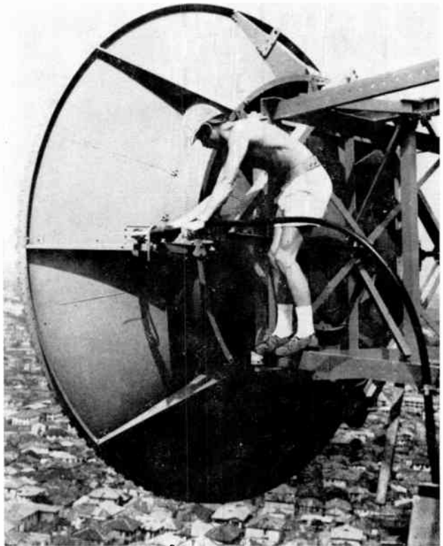
Final adjustments being made to a 6 GHz antenna at Ibadan, one of the 100 radio stations supplied and built throughout Nigeria for the 2500 mile nationwide microwave-radio trunk transmission network installed by GEC Telecommunications Limited.
