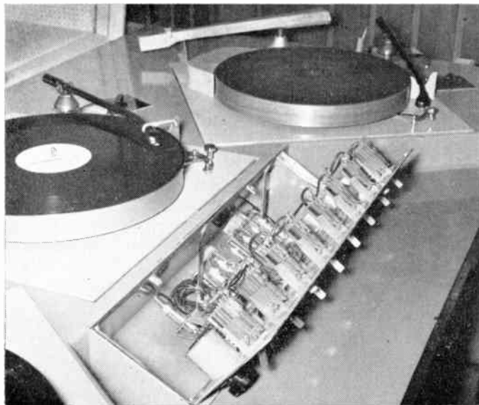
Fig. 12.—Studio control panel with key and relay panel swung forward.
