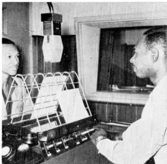
Fig. 13.—Control panel in main continuity studio.
