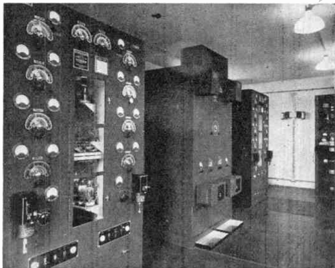
Fig. 9.—Medium Frequency Radio Range station showing duplicated transmitters. The R.F. keying equipment and coupling goniometer are housed in the unit between the two transmitters
