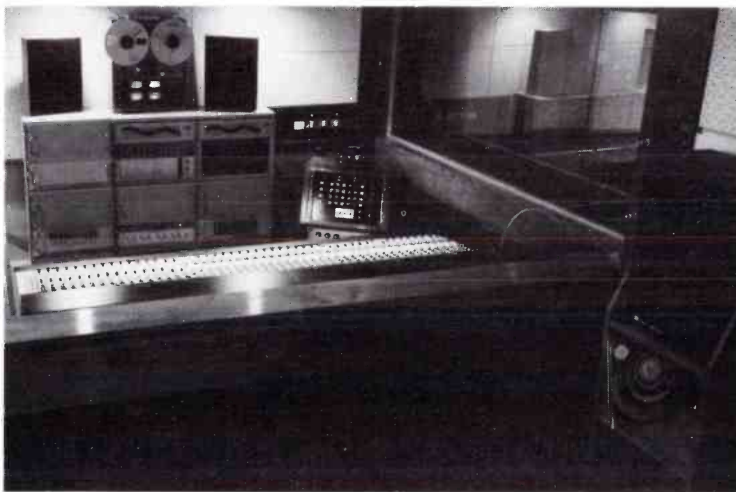
▲ Control Room with custom Allen & Heath dominating.
