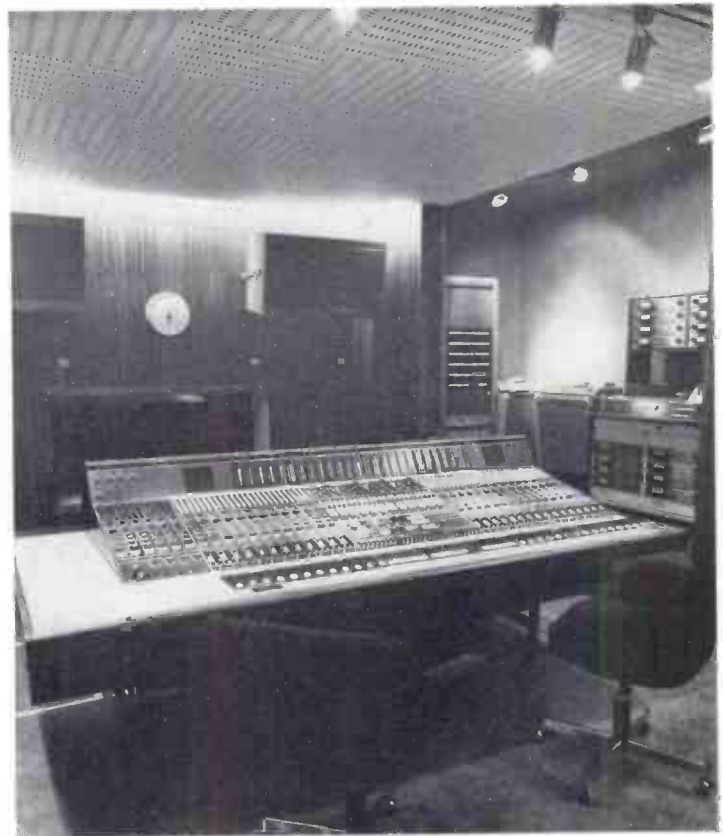
The new 24 track desk installed in Control Room A of Wessex Sound Studios, Highbury, showing the additional vocal studio in the background. This is the 24 track desk specially designed by Rupert Neve, and the only one of its kind in the world.
