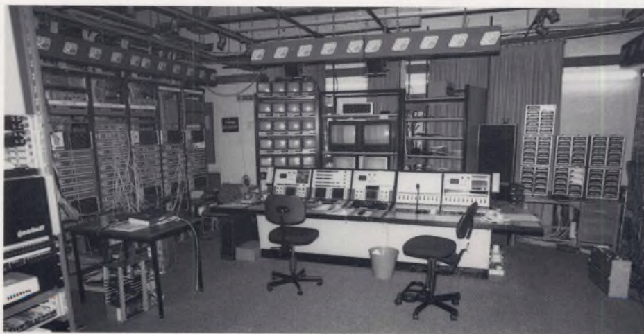
CTA control desk during the working-up period.
