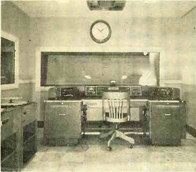
FIG. 7. THIS CONSOLE IS DESIGNED FOR THE CONTROL OF TWO STUDIOS
