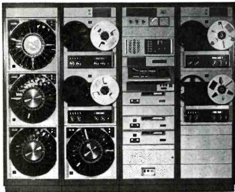
Fig. 1-5. Program automation systems increase the station's complexity and maintenance. Shown is a major program system by Systems Marketing Corp. (Model 3060), using a sequential programmer.
