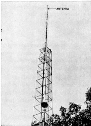
Fig. 2 — The high-band antenna mounted above the WNBW Superturnstile.
