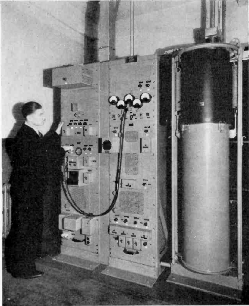
Fig. 4—Front view of a relay transmitter.
