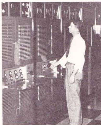
Melvin Matthews — transmitter engineer — is shown at the controls of the main transmitter. Melvin's hobby is wood working.
