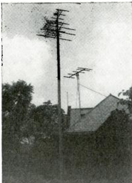
This Workshop Associates array, 90 feet in the air, is the antenna of Elmer Taflinger.
