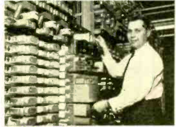
Glenn Horning, Local Equipment Supervisor, Western Reserve Telephone Company.
