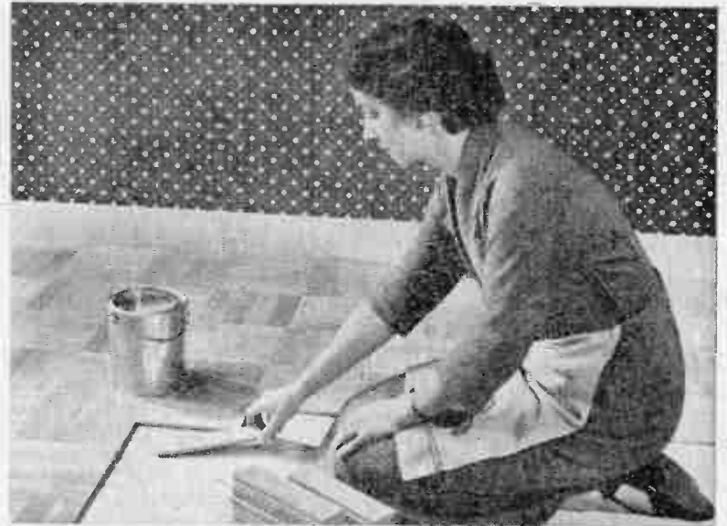
Do-it-yourself enthusiasts can lay their own parquet flooring with the aid of ready cut and machined oak blocks, special glue—and full instructions
