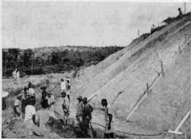
A test bank of local clay—needed for the water-imperious core of the dam
