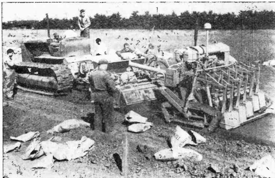
A tractor-drawn train of machines which mixes and lays a soil-cement road base as it goes along
