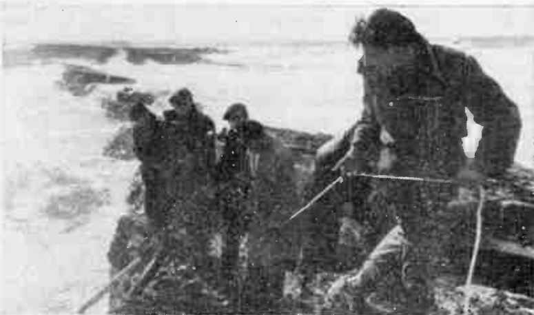
Laying pipes to carry the dangerous radio-active waste well out into the sea
