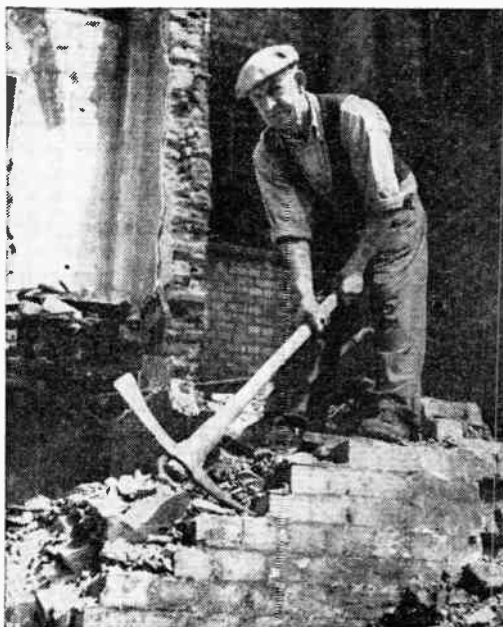
One of the workmen engaged in demolishing 100, Sidney Street, Stepney, witnessed the famous siege
