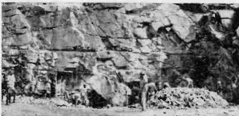
Blasting operations at Ajena to test the rock's suitability for building the dam
