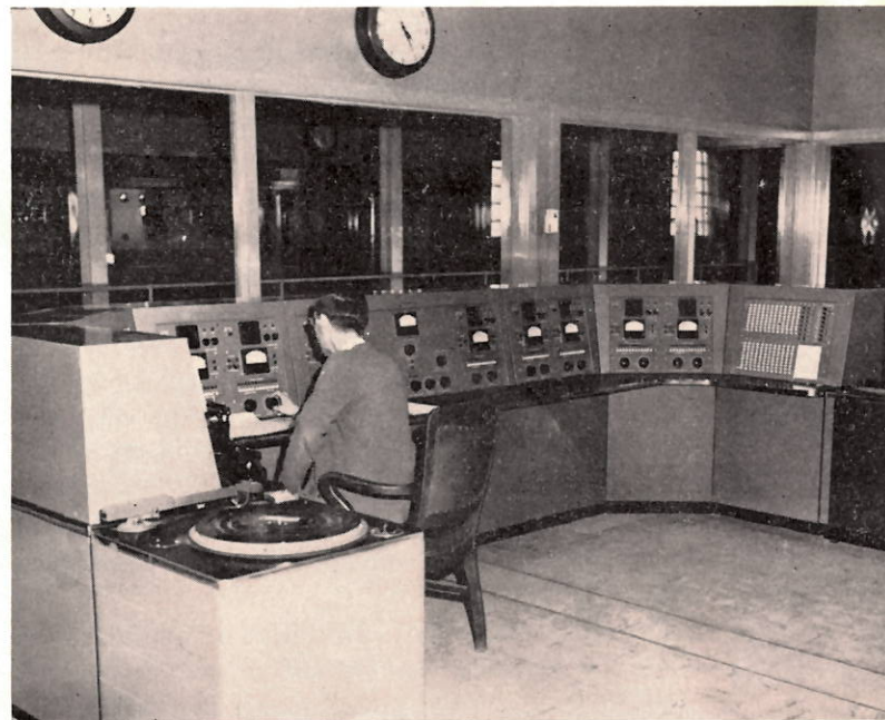
Figure 4—Transmitter control room with master control console in an overseas relay station.
