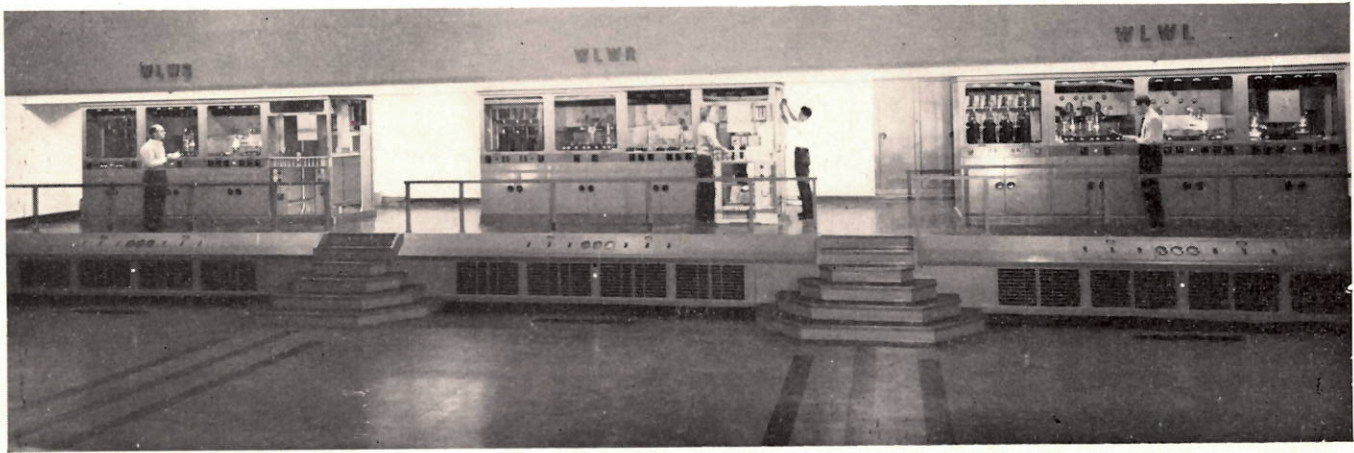
Figure 2 — View of typical VOA transmitter facilities at a short-wave station in the United States.
