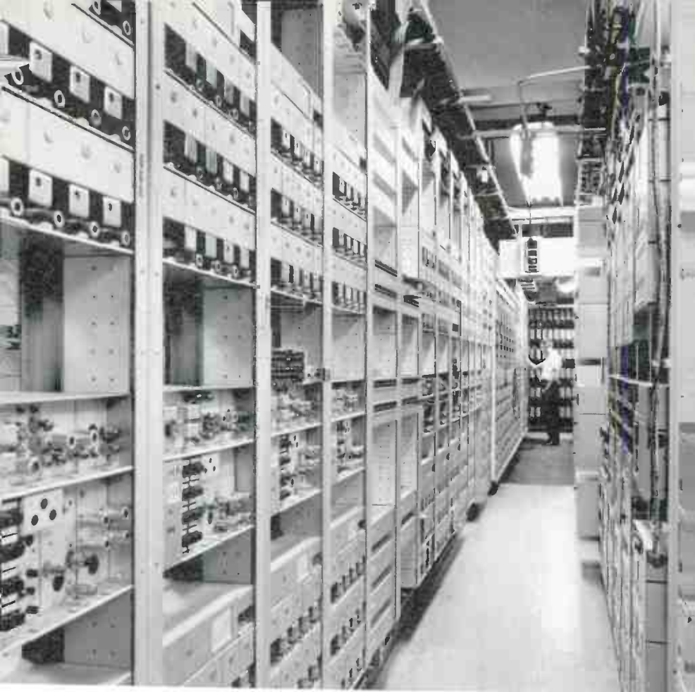
Figure 1. Lenkurt 45BX carrier equipment in telephone toll center. Protruding equipment on right is Lenkurt 33A carrier, a classic older design still in great demand because of its reliability and performance. Relatively controlled environment in such centers reduces an important problem forced on military equipment.
