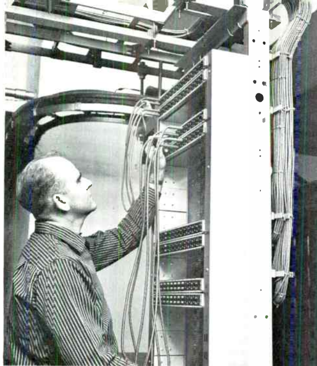
Figure 6. Typical HF or carrier frequency patch panel in telephone toll office. Shielded twisted pair is used to minimize coupling between adjacent circuits.
