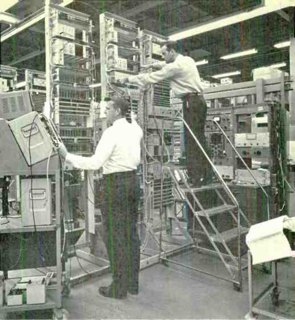
Figure 1. Quality assurance engineers perform complete system performance test on Type 46A carrier equipment, before shipment to customer.
