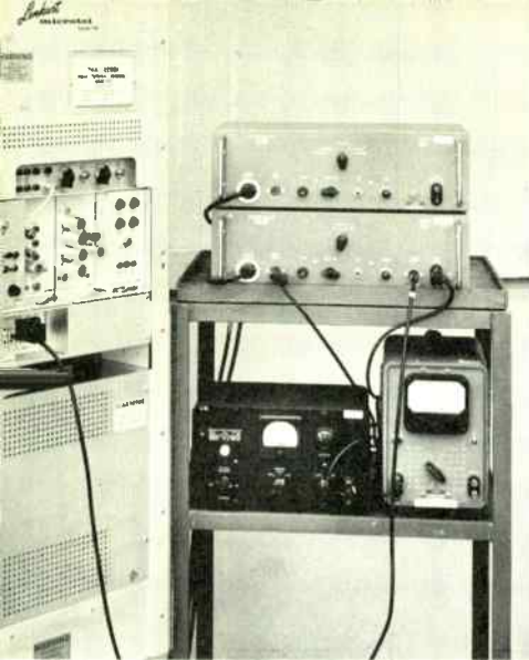
Figure 4. Lenkurt Type 5203-5204 Distortion Test Set in use. This equipment works on principle diagrammed in Figure 3.
