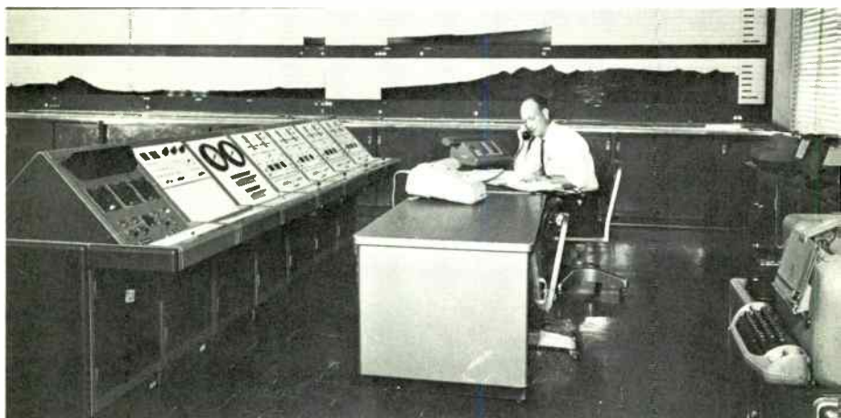
Figure 5. A typical centralized control station for a pipeline. From this location are monitored such operational details as flow rate, pump pressure and suction, fluid viscosity, and the like. Distant operations can be adjusted in response to changing loads and other variables. Panels in background show profile of terrain which pipeline traverses, and which has important bearing on operating parameters. Centralization is made possible by efficient digital transmission.
