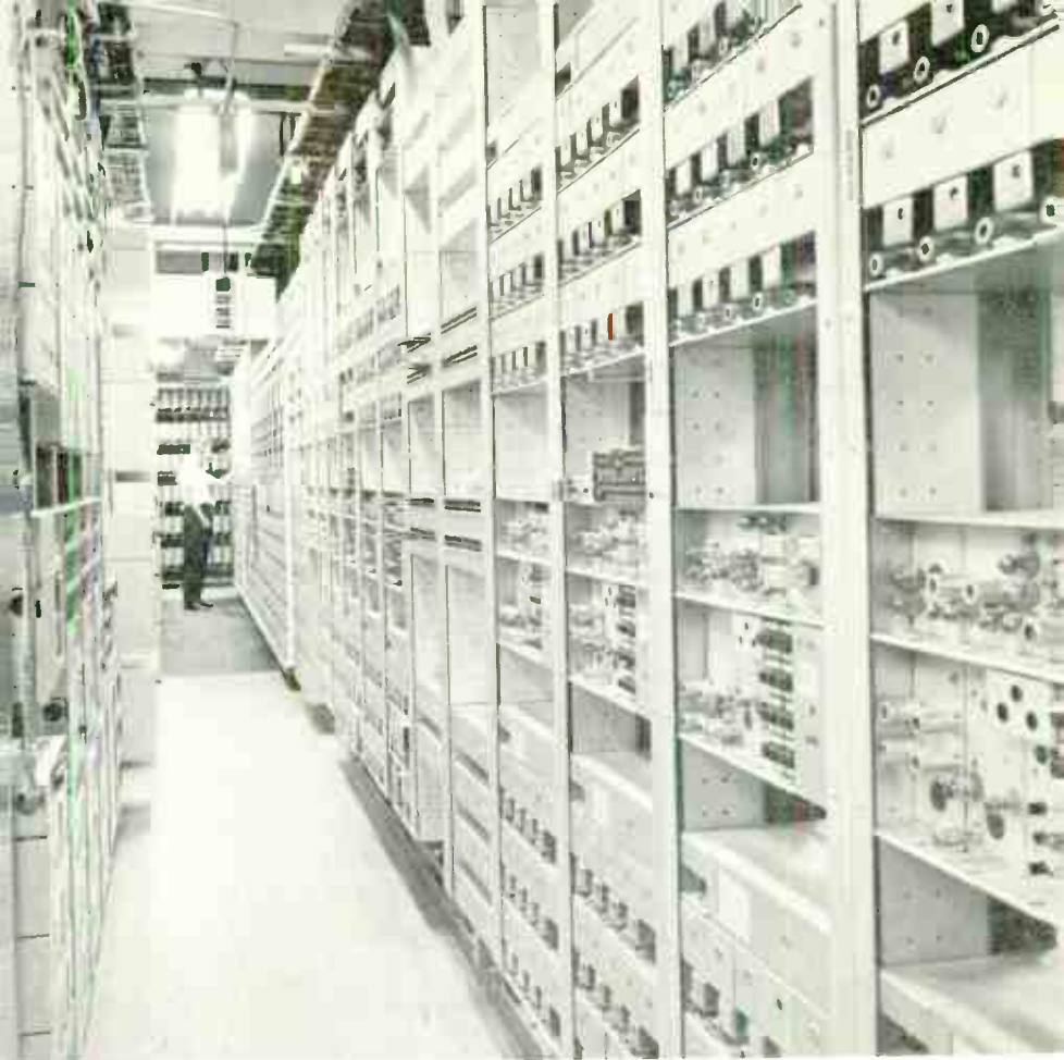
Figure 1. Carrier equipment like shown above enables hundreds of channels to be transmitted over a single radio beam. Increasing traffic density makes it imperative that some sort of standby protection be provided for microwave equipment.
