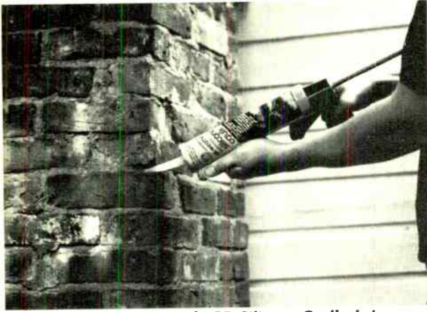
Amazingly tough GE Silicone Caulk, being used here to repair a brick chimney, will also repair wood shingles or concrete walks.
