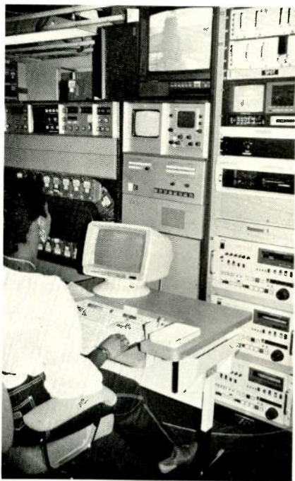
WPIX engineer Sheryl Leito uses the SPOT automation system, right rack, to copy quad material from the cart machines at her left onto BVW-40s.
