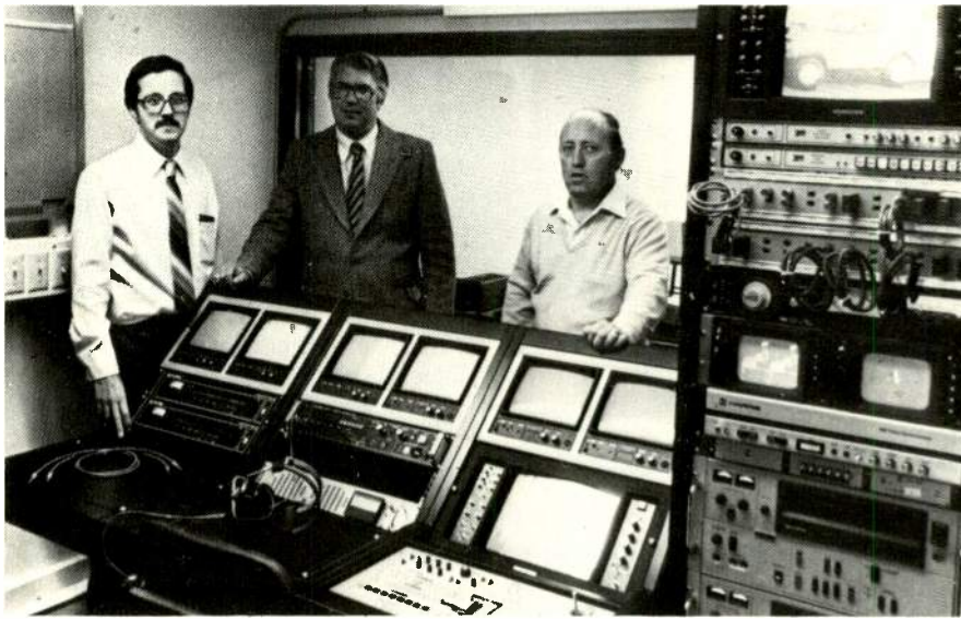
Montgomery Publications' LPTV station K6KZ in Junction City, KS recently completed equipment installation with video systems design by Lines Video Systems.
